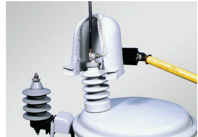
4. Extend the hotstick to the necessary length and apply the guard, taking care to position the trigger between the top and second bushing sheds.
